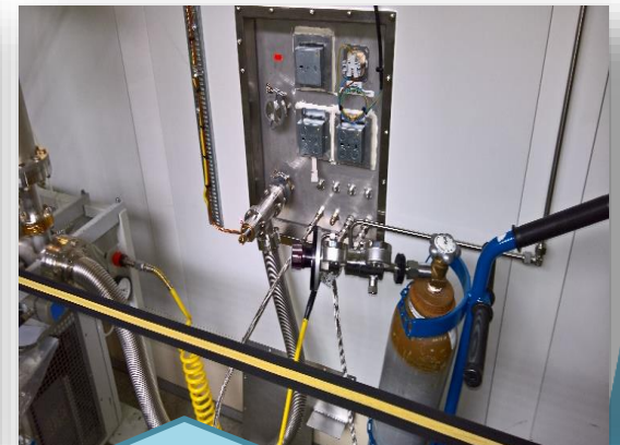
Panel outside clean room
