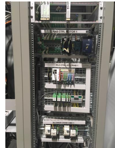
Control rack for Cavity 1
