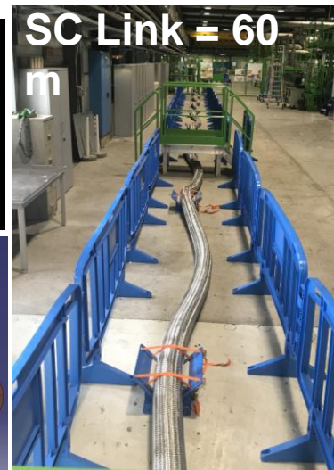
Un-shielded cryostats validated
