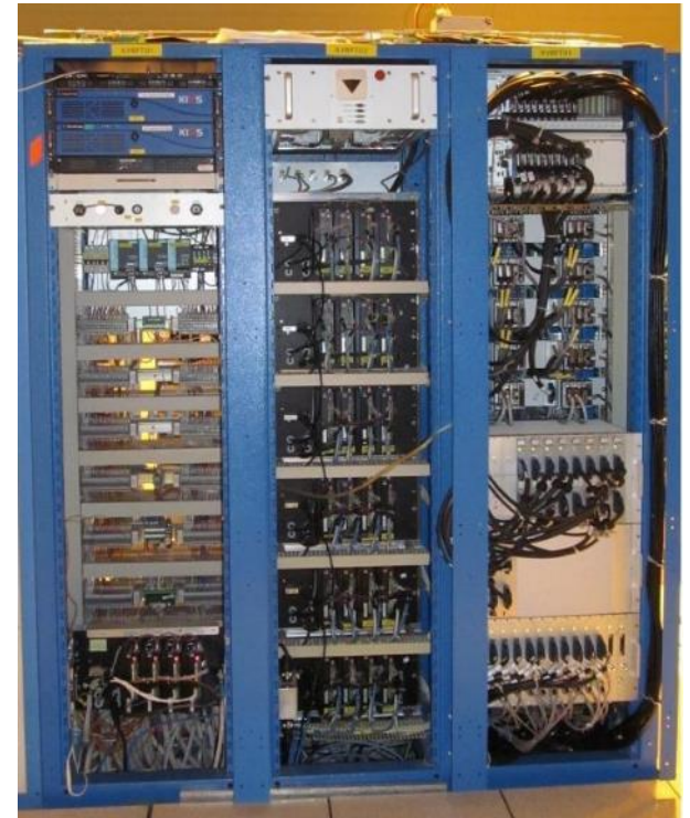
Totem Position Control Racks
