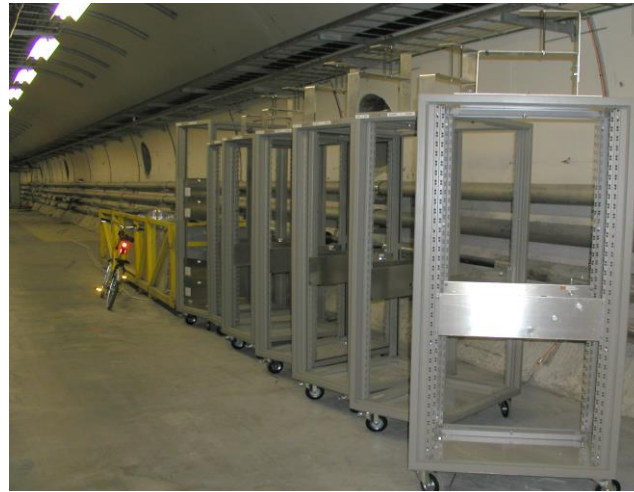
Mockup power converters (LHC installation)
