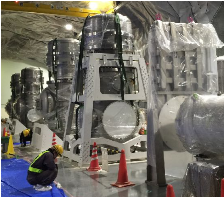
Vacuum chamber for BS Achieved pressure 10^{-5} Pa
