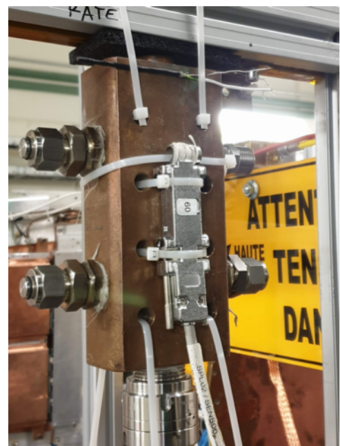
EN-CV - tightness of cooled cables manifolds
