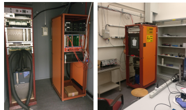
Test racks for the commissioning
