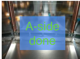
FC HV infrastructure modification
