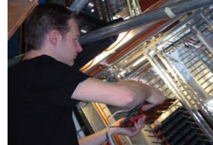
Install new FEC + test
