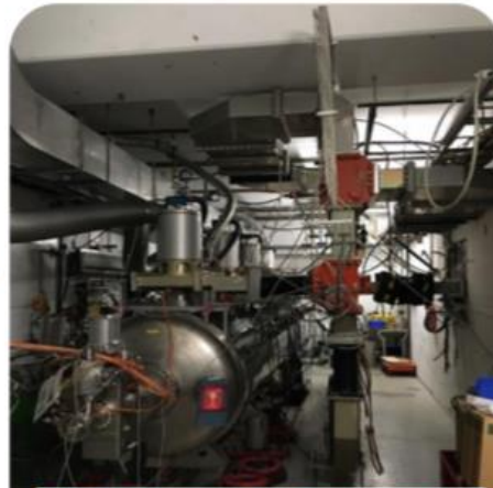
CM installation and RF Test
