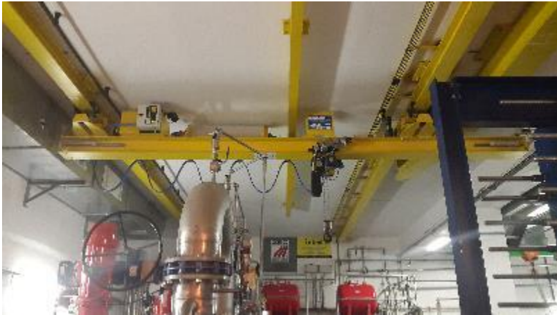
Underhung cranes in underground cavern USC55
