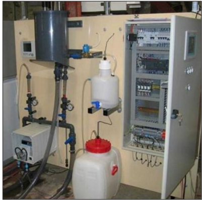
Water Monitoring Station (x7)
