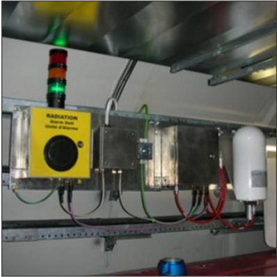
DA Monitoring Station (x142)
