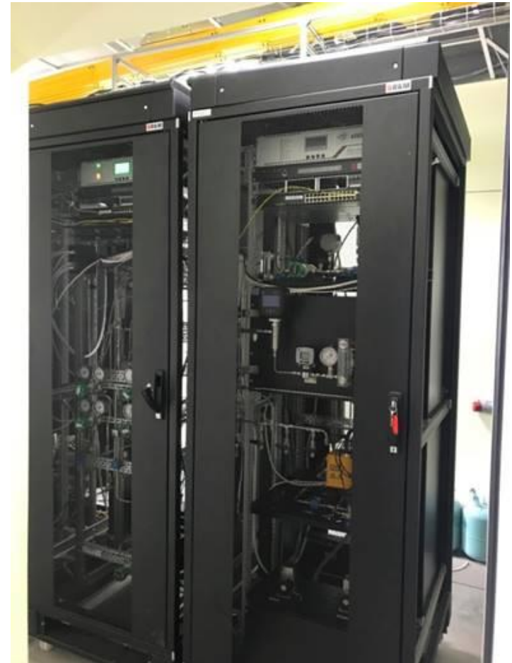
Racks for Slow Control electronic equipment
