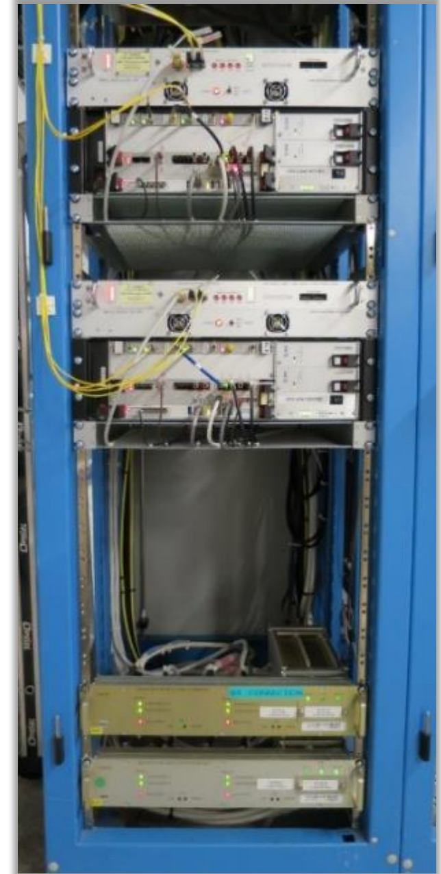
BCCM installation in UA47
