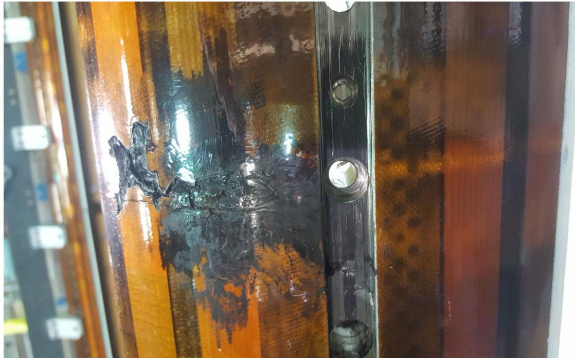
Electrical short circuit in MQXFAP1 [G. Ambrosio, et al.]
