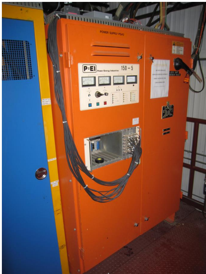
150 kW Power Energy Industries (PEI) PS module
