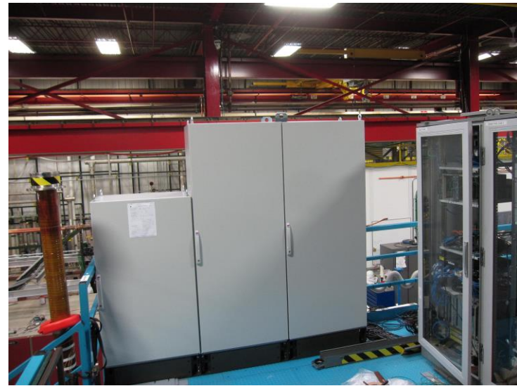
New PLC cabinets at TS4
