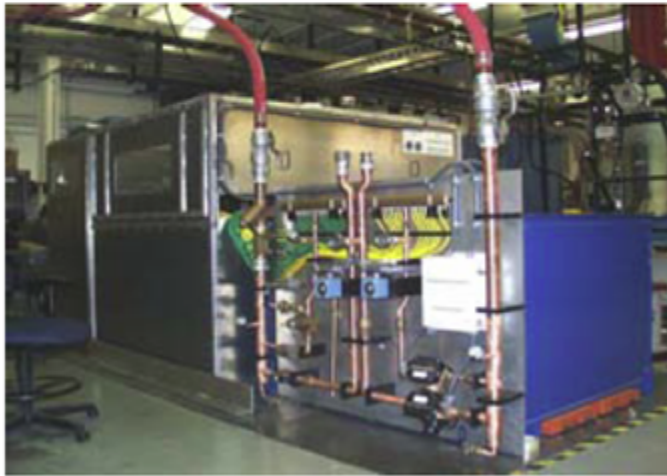
High Voltage Converter Modulator
