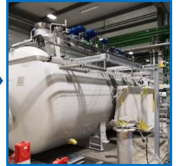
Cold Box installed 2019 MAY, 15
