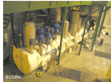
Distribution Valve Boxes
