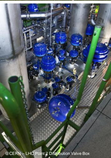
@CERN – LHC Point 2 Distribution Valve Box
