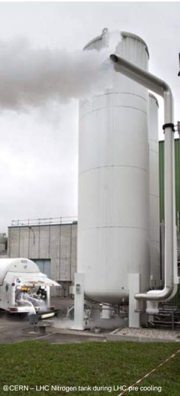
@CERN – LHC Nitrogen tank during LHC pre cooling
