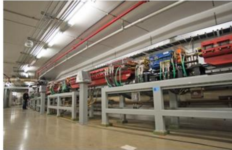
A view of the APS BOOSTER
