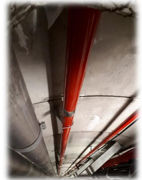
Dry riser in Shaft 1
