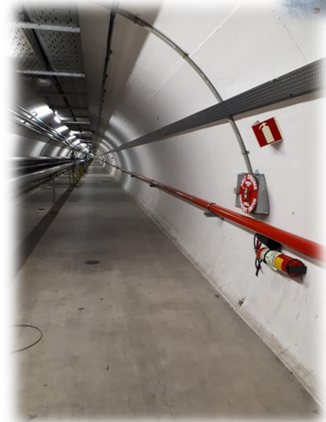
"Goulotte", dry riser and new fire extinguishers in TT10
