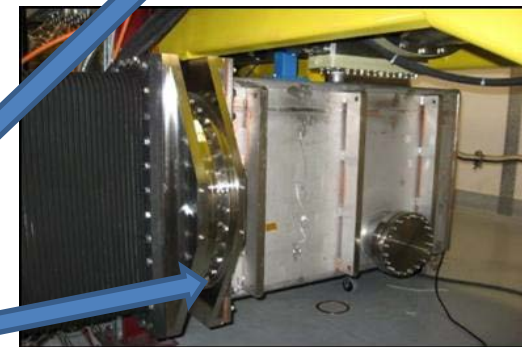
Two Cu coated SS WR 2300 waveguide power couplers installed in the DTL/CCDL in LINAC 4 tunnel at CERN
