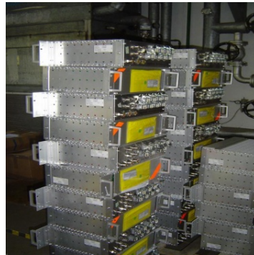
nQPSRacks ready for installation
