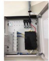
New optical fiber @ server room
