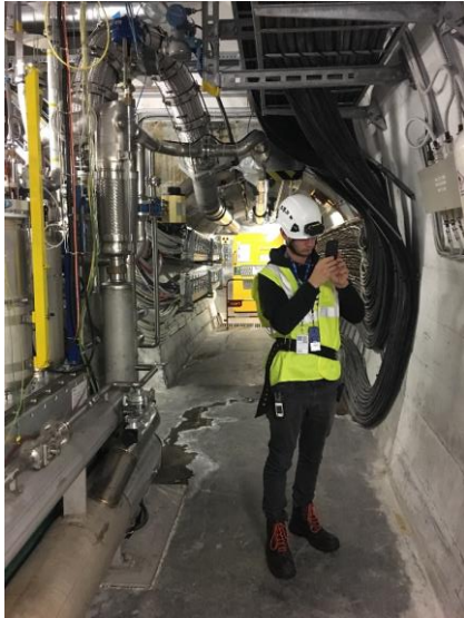
Faults recorded on a mobile app (TIC)
