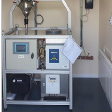
Ventilation Monitoring Stations (x10)
