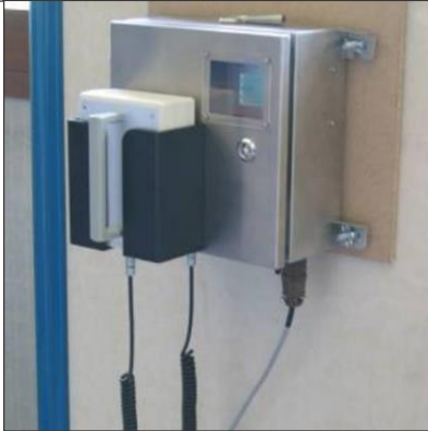
Material Control Monitor (x19)
