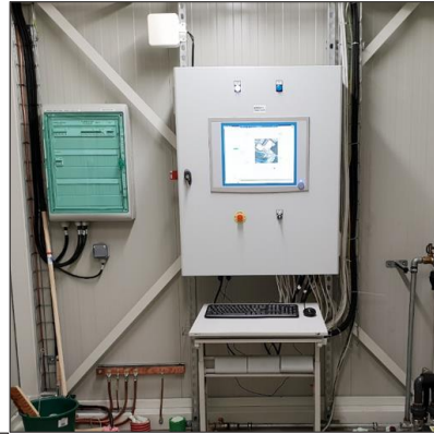
SMART Water Monitoring Station (x6)
