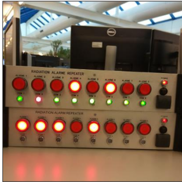
Alarm repeaters (x28)
