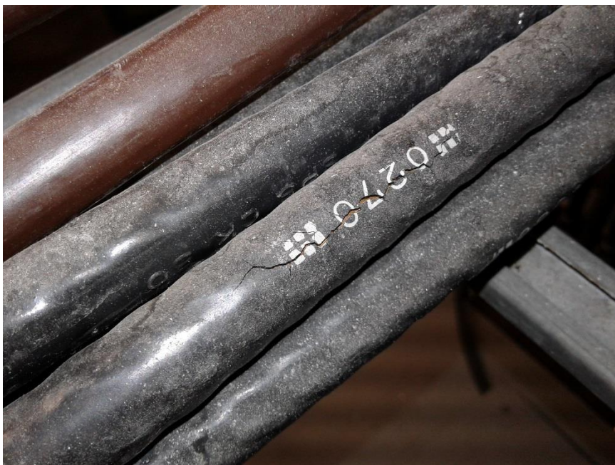
Insulation cracking on a cable going to R21B.
