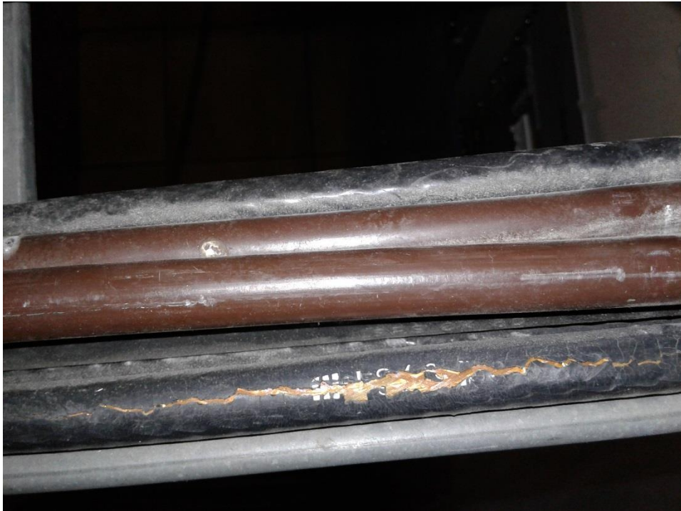
Similar degradation shown on a cable to R22A patch.
