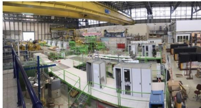
CERN: Test facility completed for the Super-FRS s.c. dipoles and multiplets
