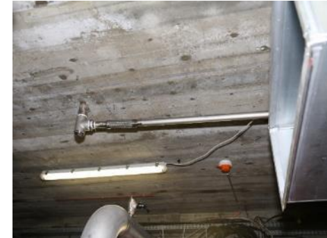
Collector pipe at lowest point of floor
