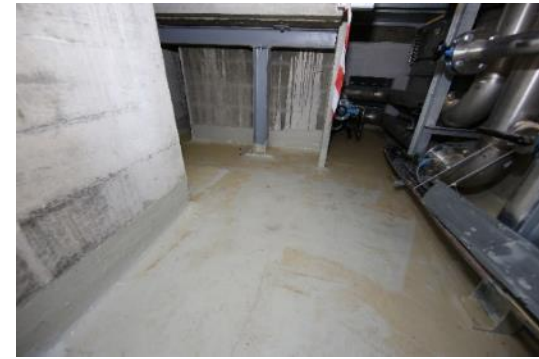
Retention tank 2: 1900 L
