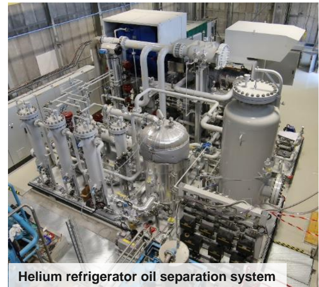
Helium refrigerator compression station
