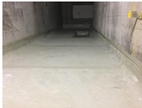
Retention tank 1: 1900 L
