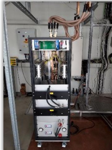
System under test in MPE lab.
