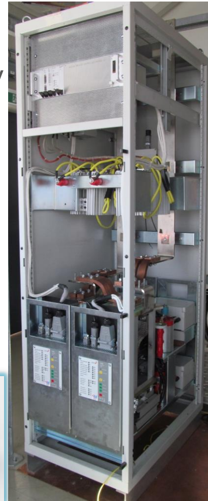
2kA EE system
