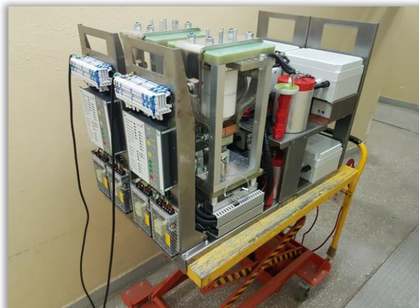
Two vacuum switches built in a sliding cassette
