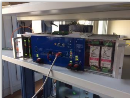
3U control chassis housed the electronic boards
