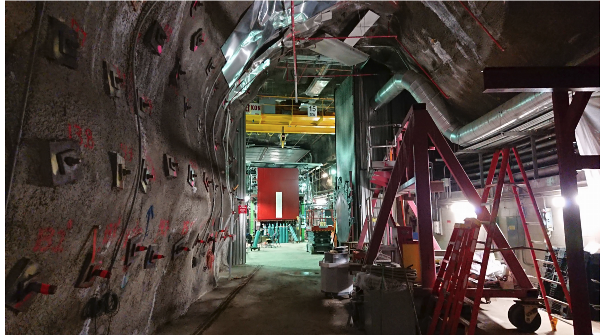
MINOS-ND hall at Fermilab.
