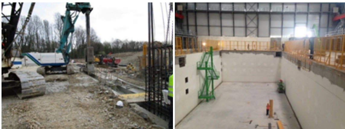
Fig. 36: Photographs taken during (left) and after (right) diaphragm walling works at CENF.
