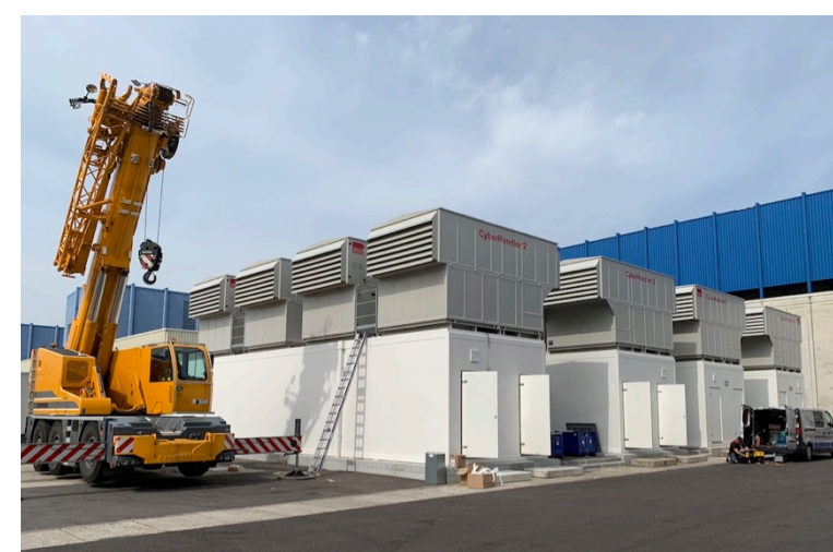
Containers for O 2 system
