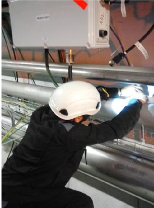
Cabling Minirack – Boxes containing old electronics.
