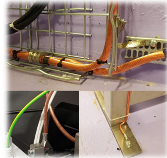
Grounding by LHCb
