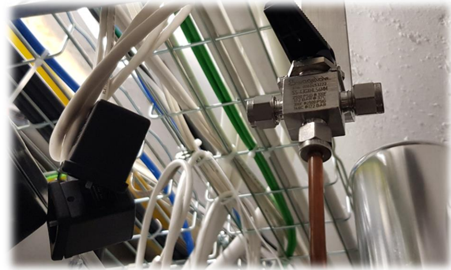
Last sensors (PT and TT) for main chiller
