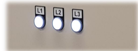
Power distribution EN-EL
