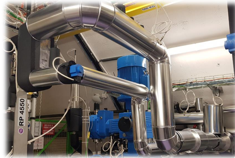
Piping and insulation
