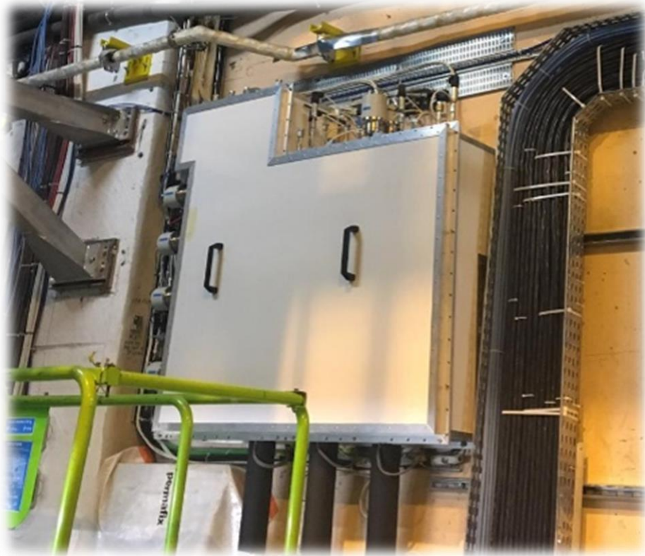
Bypasses for Distribution Boxes simulation and connection to transfer lines
