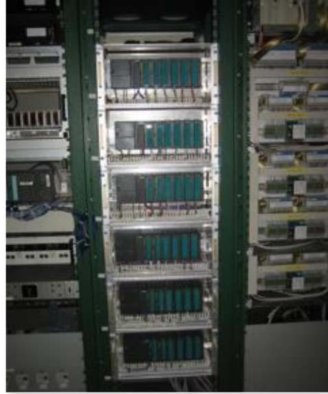
Control system PLC based
