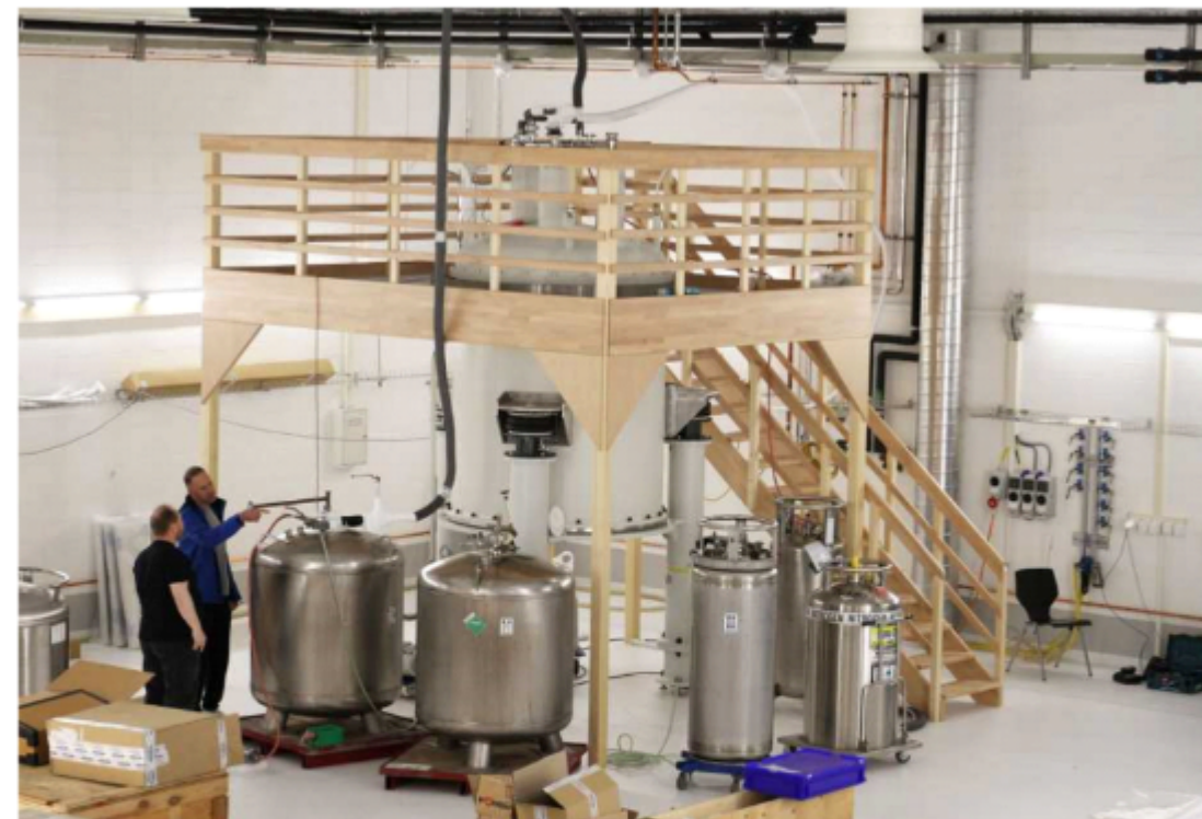
The Bruker Ascend 1.2GHz NMR installed at the ETH (Zurich)
