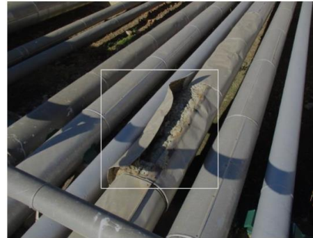
STEEL PARTIAL DETACHMENT
