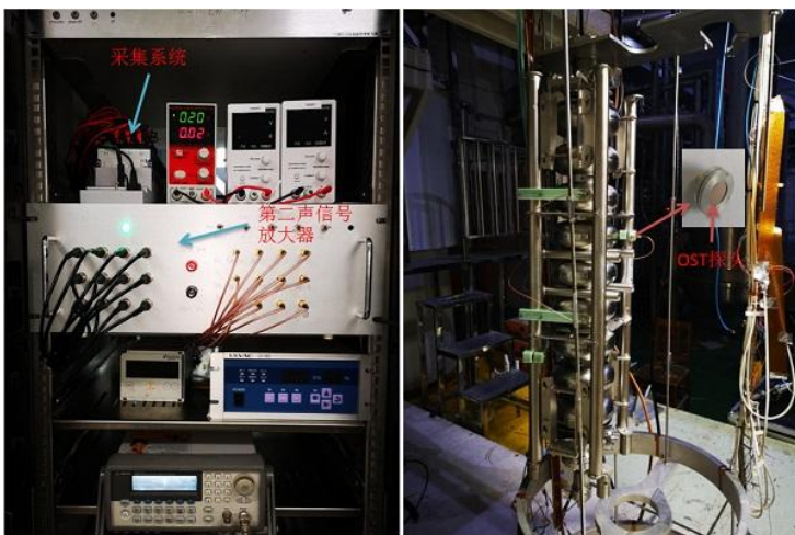
SC cavity vertical test temperature monitor system established
