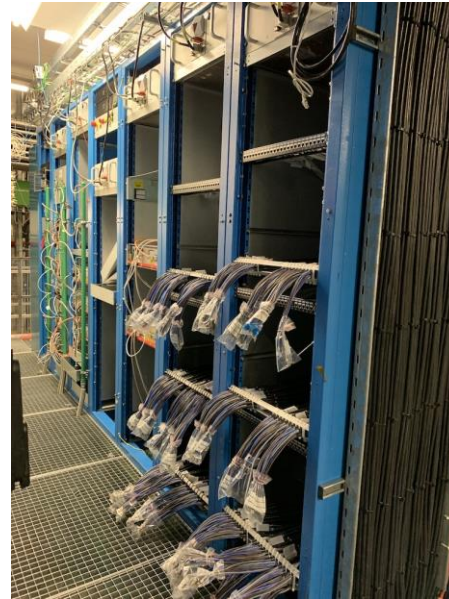
ITS racks A12-13
