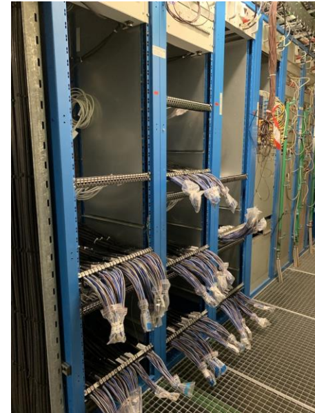
ITS racks A07-08-09
