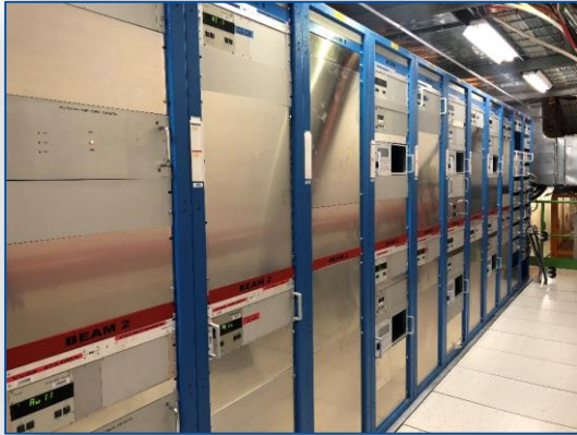
LSS5: LS2 Vac. Controls Rack and DP Cons.
