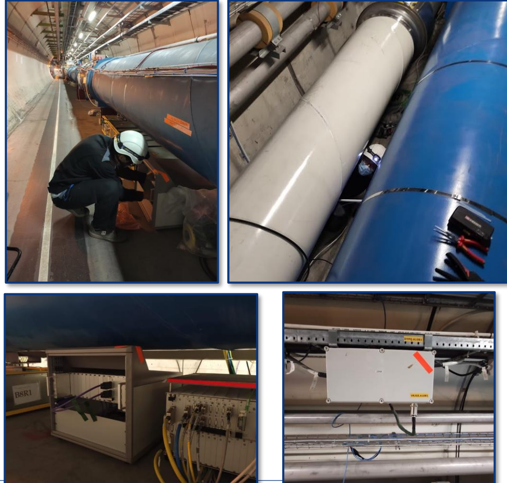
R2E Installation ARC12
