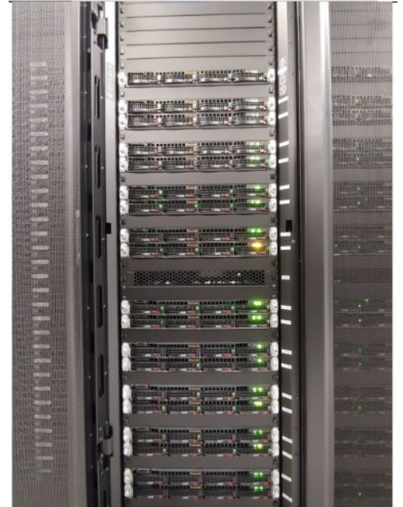
Rack of Supermicro SYS-6019TR4 Servers
