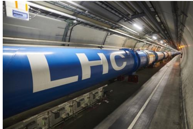
The LHC tunnel. Image: CERN
