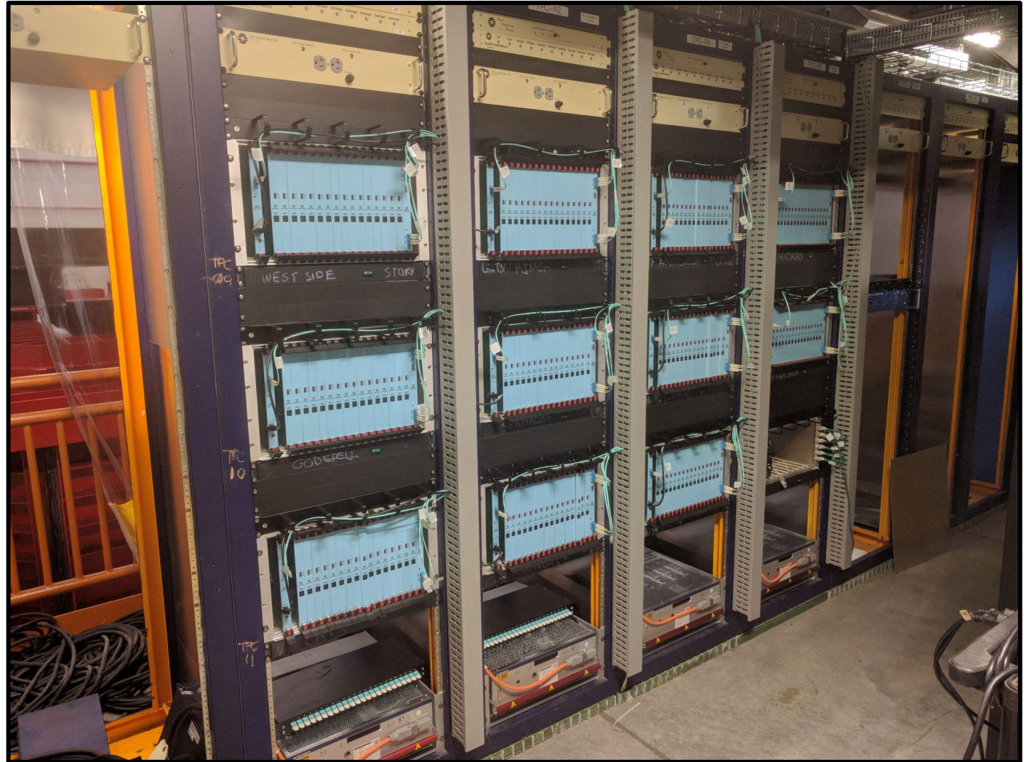
Data Acquisition System electronic racks installed in the mezzanine level, February 2020
