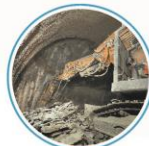
CIVIL ENGINEERING 2 new caverns, 1km underground galleries, two new large shafts; 10 new technical buildings on surface in P1 and P5 (near ATLAS and CMS)
