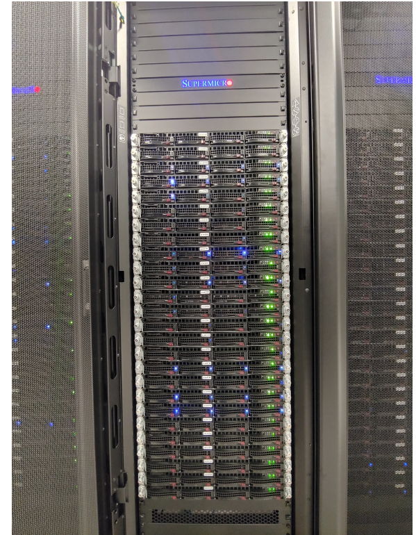
Rack of new EPYC-based Supermicro 1023US-TR4 Servers
