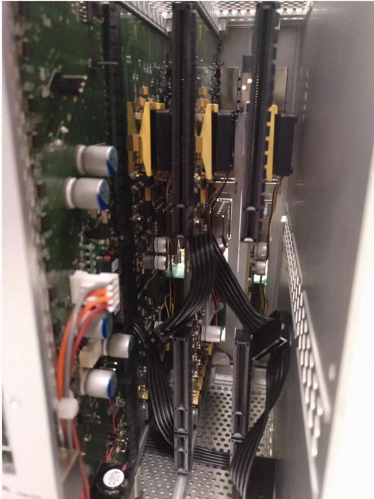
2 FECs and FEC with DVMM SATA cable for all DVMMs in place
