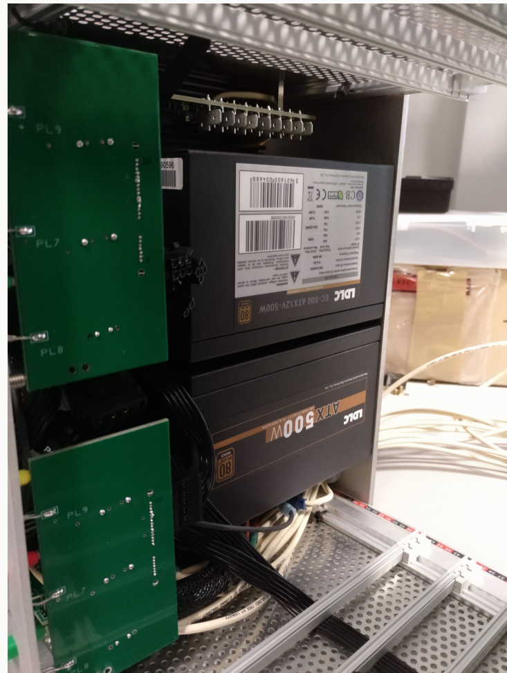
ATX power supplies AUX monitor cards
