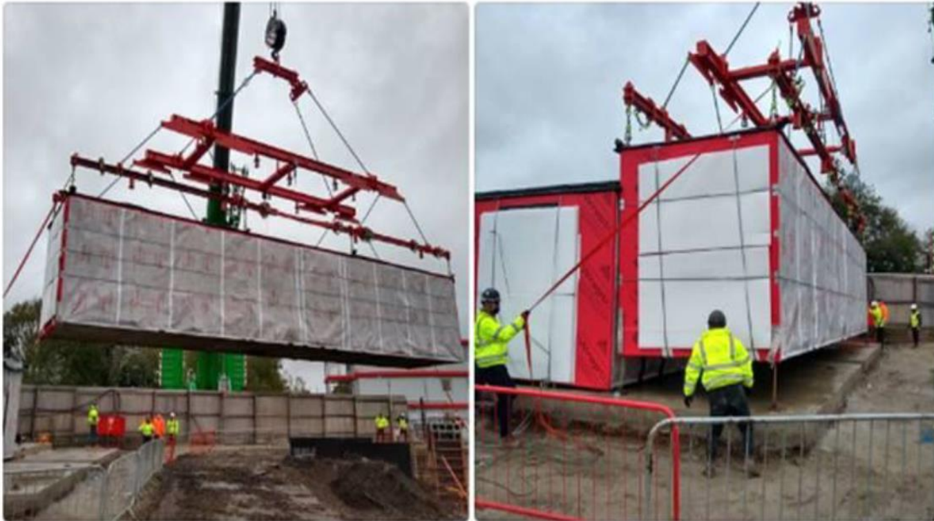
Modular prefabricated housing Isostatic concept to control forces on lifting points Canturbury (UK) – Nov, 2020
