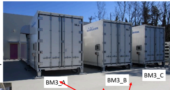
Capacitor Banks for BM3
