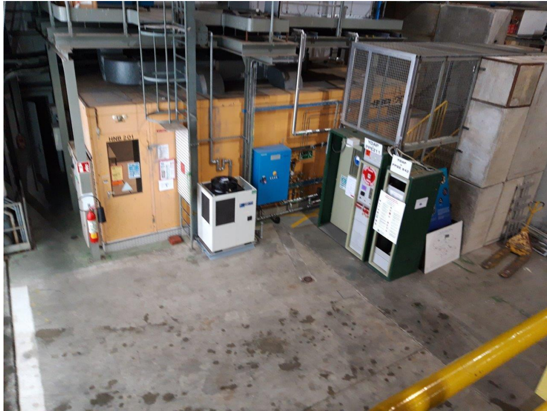
“Bellegarde side” entrance door; available area shown in the picture is sufficient
